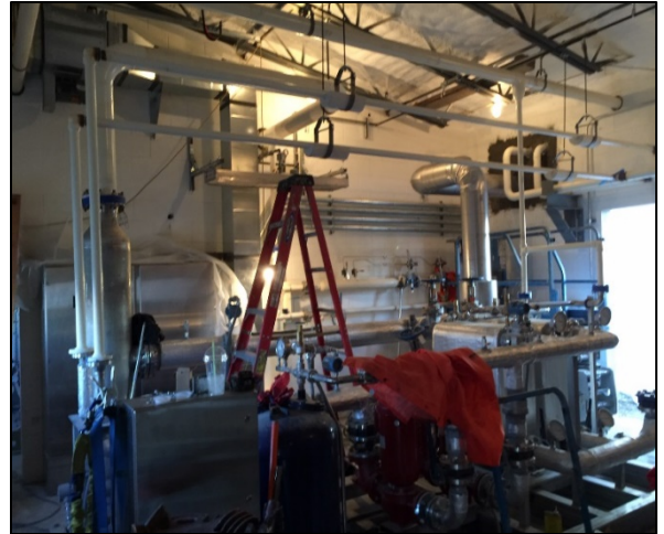
Boil-off Gas Heater
