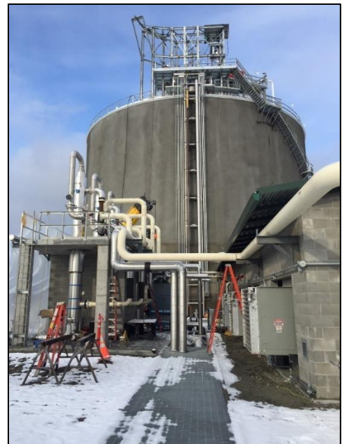
Balance of Plant Piping
